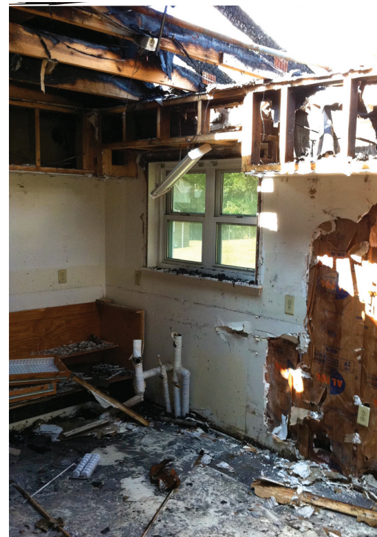
FIRE AND SMOKE DAMAGE TO WILLOW VALLEY COURT UNITS IN COOKEVILLE DUE TO FIREWORKS.
